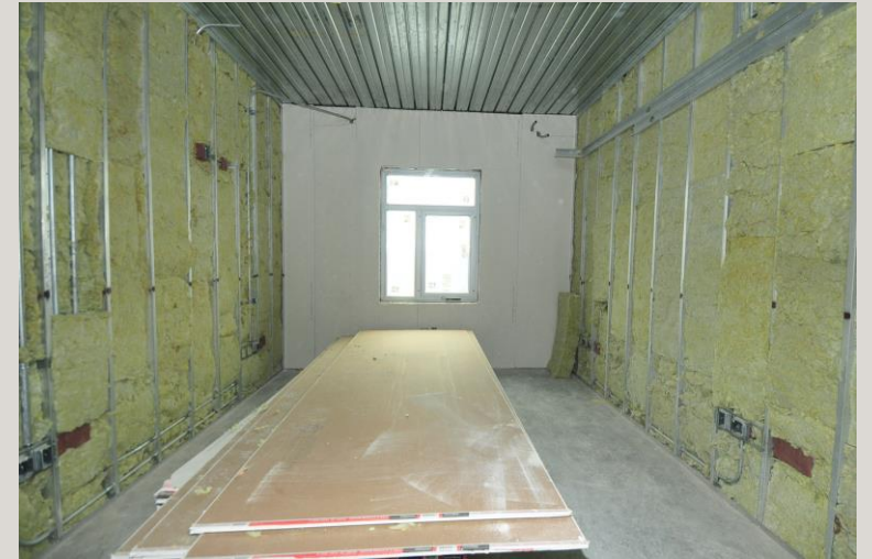
Typical Bedroom with Soundproofing
